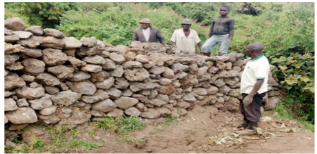
The two photos are repairs of damages caused by buffalos along Nyagakenke and Kanombe villages, MGNP
