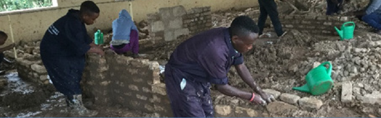
Batwa supported students during Brick Laying and Concrete Practice at African International Christian Ministries - Kabaale District
